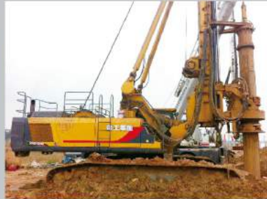
新郑机场跨航空港区南水北调工程大桥 XCMG rotary drilling rigs are working in South water to North Project
