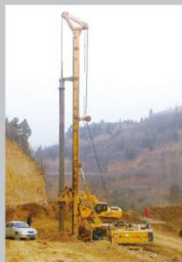
陇海路高架延伸栎阳段XR360施工快速高效 XR360 was working in Longhai railway with high working efficiency
