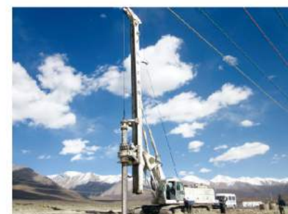
XR220施工照片——兰新铁路青海高原工地 XR220 was working in Lanzhou-Qinghai railway in plateau
