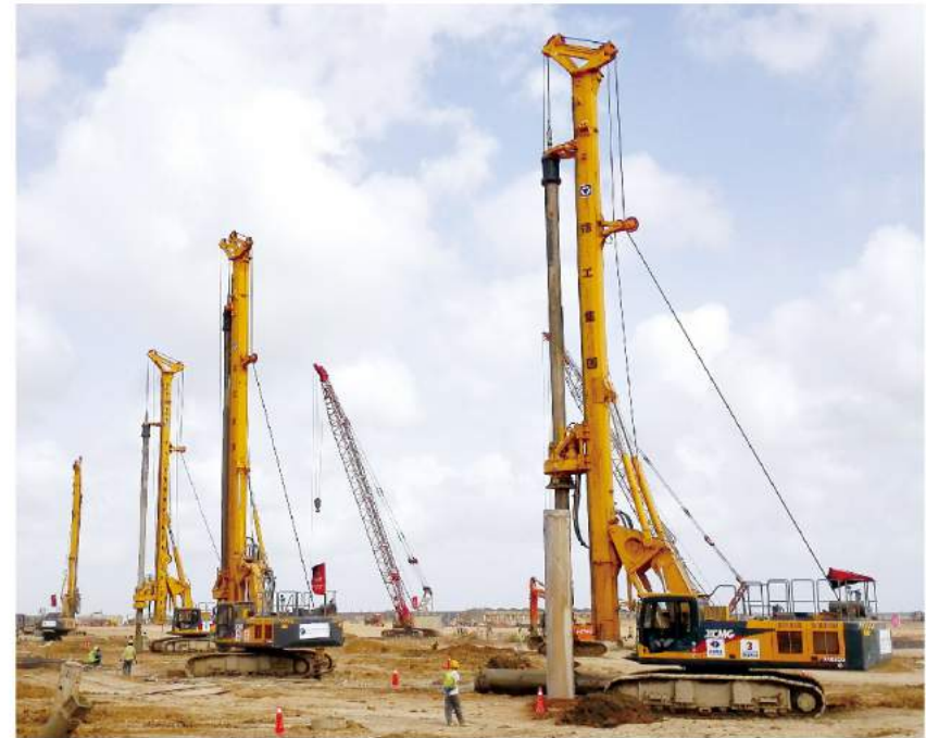
徐工旋挖钻“一带一路”显风采，群机助力巴基斯坦新建设 XCMG rotary drilling rigs are working in One Belt, One Road project in Pakistan
